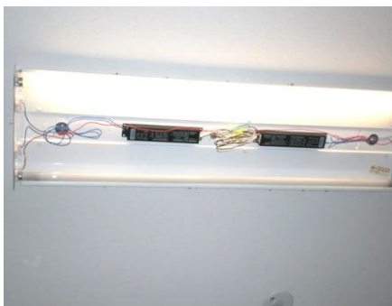
Existing electronic ballasts and 32 watt T-8 lamps in new school addition.
