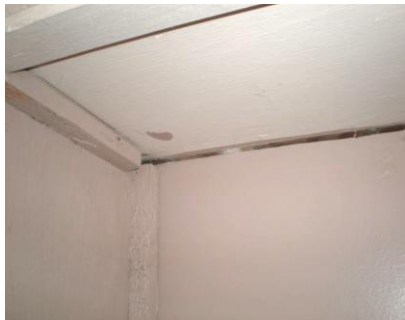
Before air sealing. Large gaps in plywood seams allowed substantial air leakage through thermal boundary
