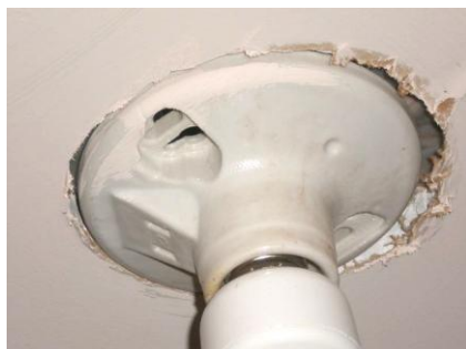
Existing light fixture. Large gaps allowed substantial air leakage through thermal boundary
