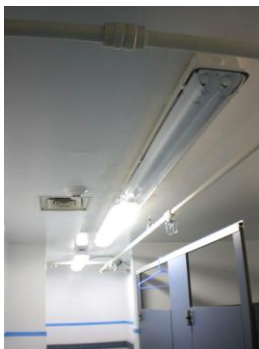
T-5 fixture taken offline in over-lit bathroom.
